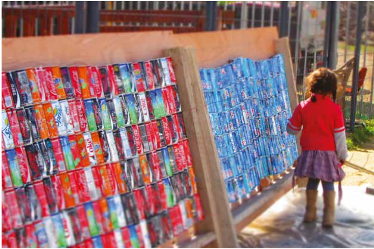
The solar heating system is constructed from used soda cans, later painted black.
